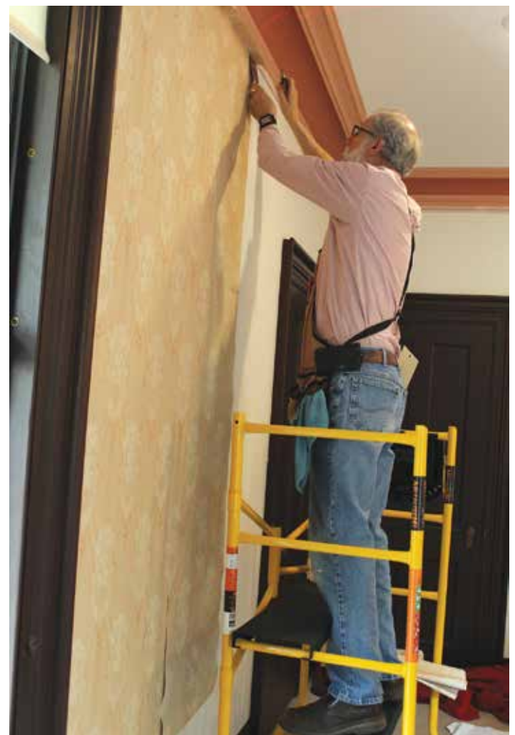
Wallpaper installation in the Stowe House Dining Room, done by Denis Picard of Kensington, CT. The paper being hung is a reproduction of a paper in the Stowe Center's archive.
